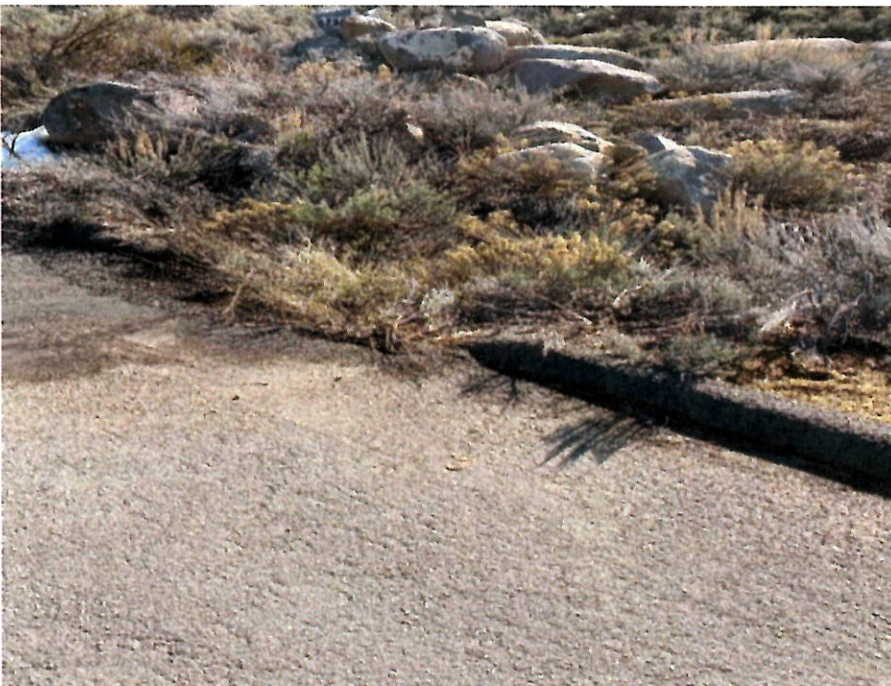
Photo 2. Gap in curb on south side of Cedarwood Drive.
