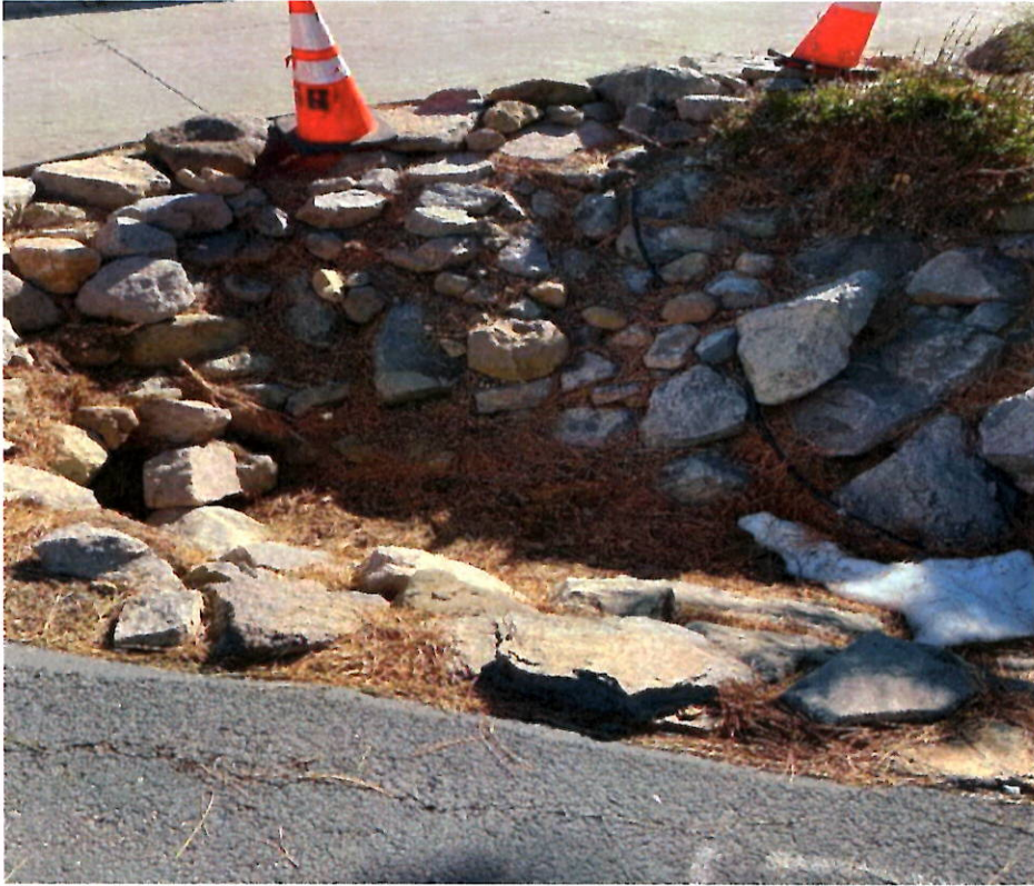
Photo 5. Outlet of culvert under Parcel A and point at which flow is diverted west under Access Road.
